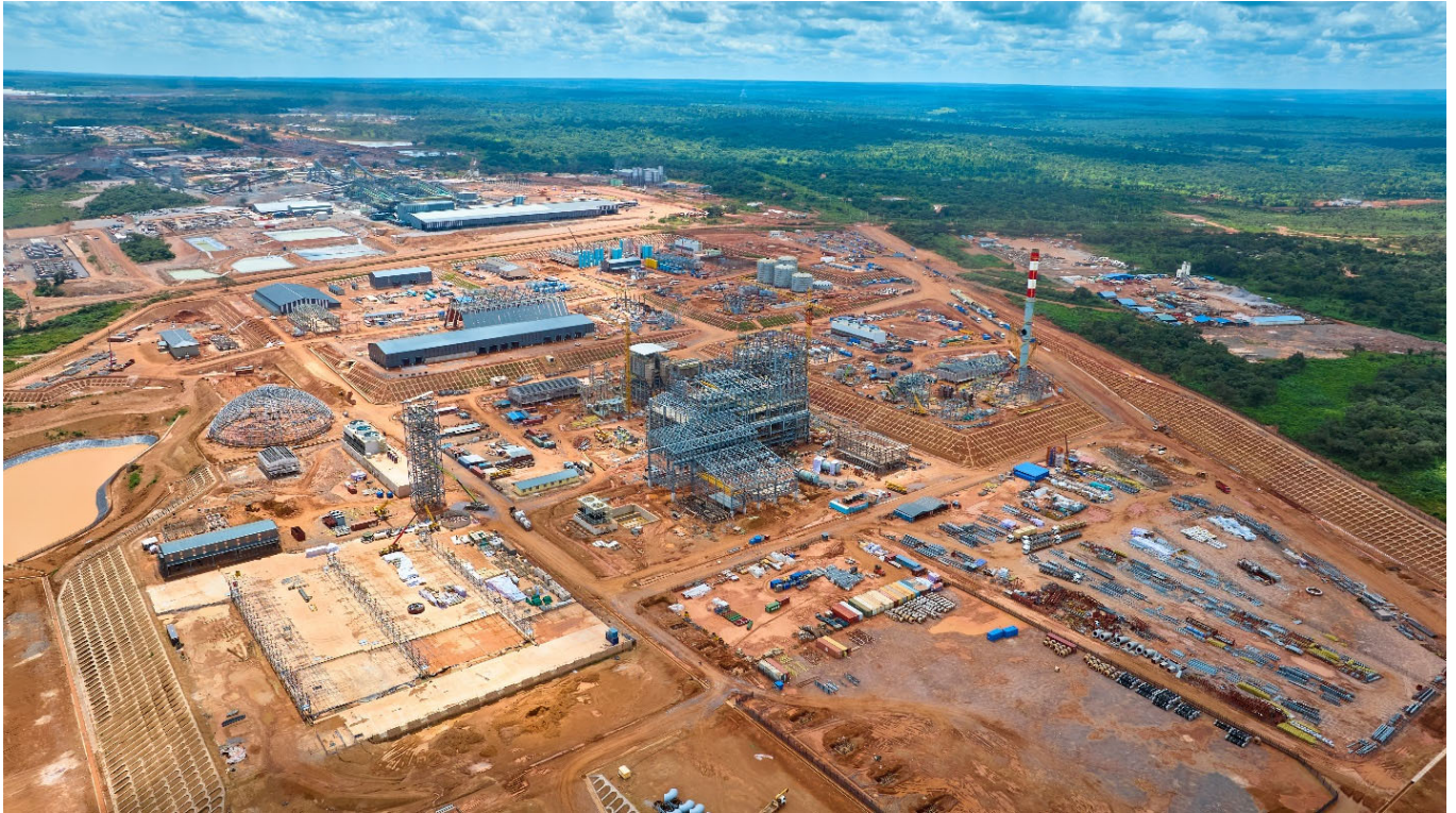
Photo: The Phase 2 smelter construction site with the Phase 1 and Phase 2 concentrators in the background. The smelter complex remains on schedule for commissioning in Q4 2024.
