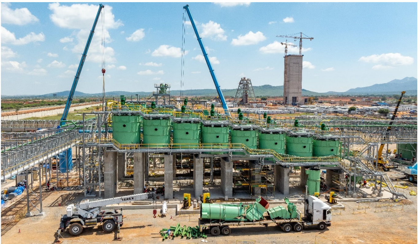
Photo: Looking north over the flotation cells of Platreef’s 770,000 tonnes per annum Phase 1 concentrator, with the headgear of Shaft #1 (left) and Shaft #2 (right) in the background.
