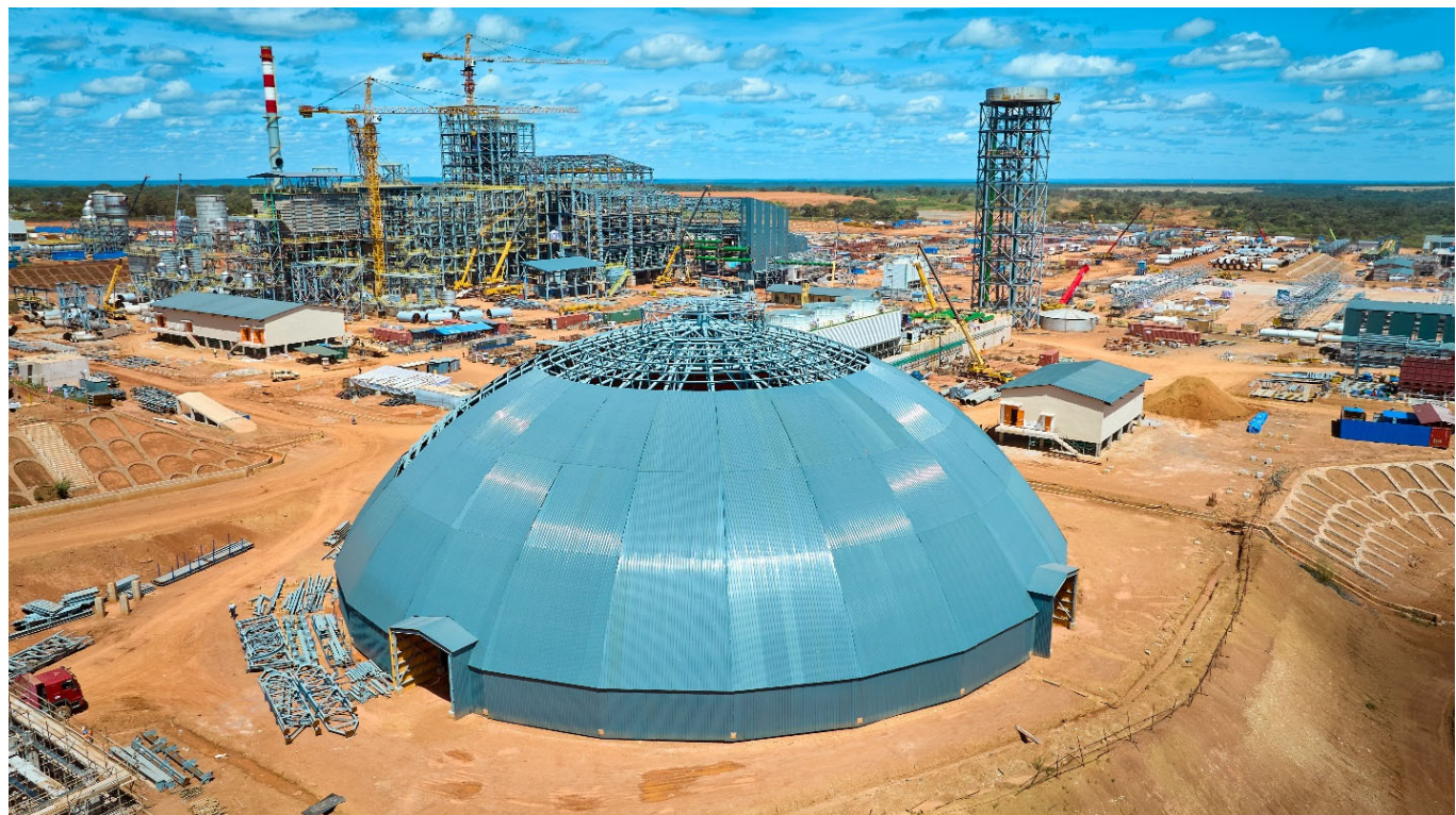
Photo: Construction of Kamoa-Kakula's Phase 3 smelter concentrate blending building. The smelter project is on track for completion in Q4 2024.
