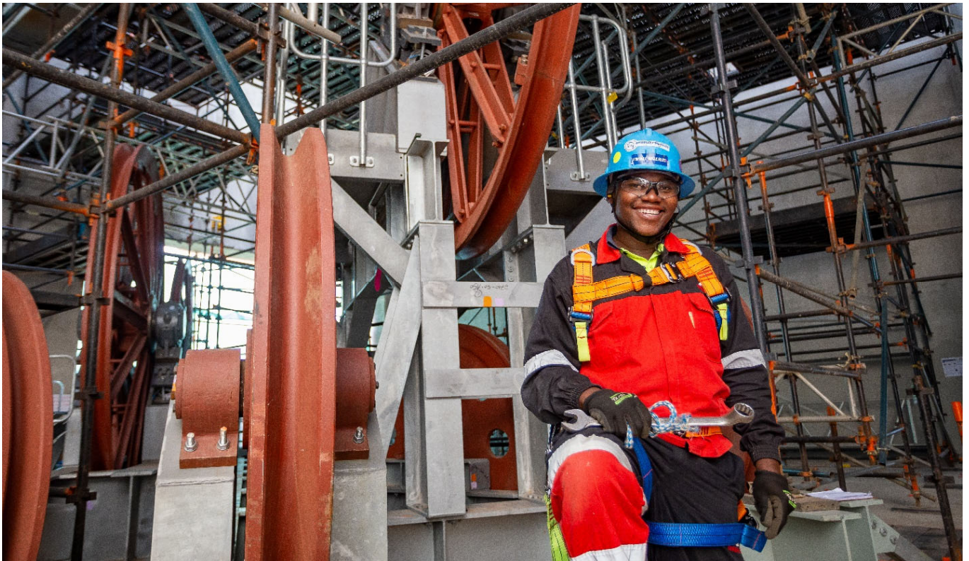
Photo: Calvin Sekele, General Worker, stands at the foot of Platreef's Shaft #2, where construction activities are advancing well on the installation of 1,124 tonnes of internal structural steel inside Shaft #2's headgear.
