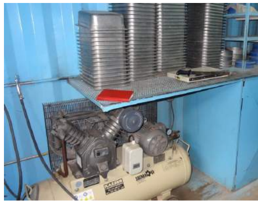
C Compressor and sample trays
